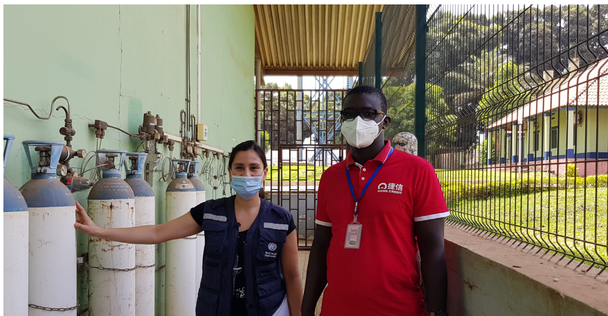
WHO staff look at current oxygen supply systems at a health center.
